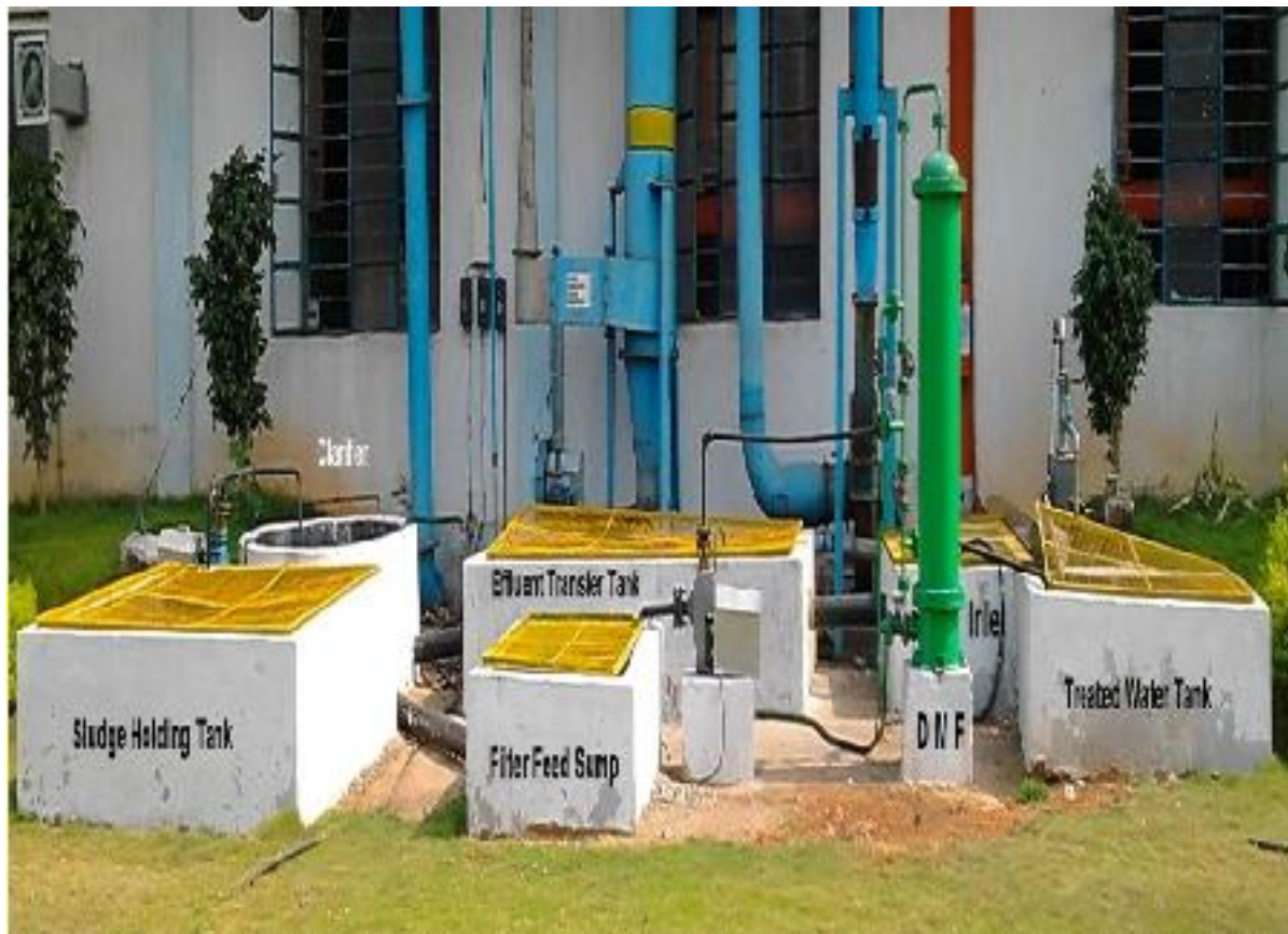
10 KLD WASTE WATER TREATMENT PLANT FOR M/s. VESUVIUS INDIA LTD, VISAKHAPATNAM
