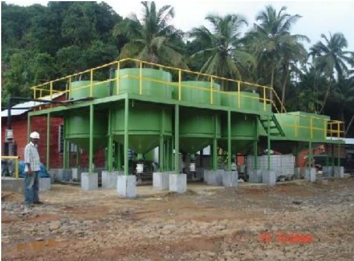
3 MLD WASTE WATER TREATMENT PLANT FOR MANGALORE CAVERN PROJECT, M/s. SKE&C-KCT (JV), MANGALORE, KARNATAKA
