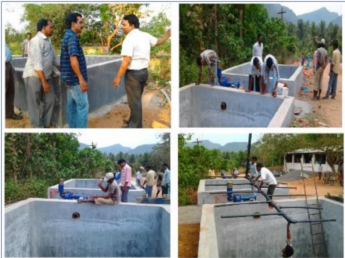
150 KLD Sewage Treatment Plant for M/s Maharaja Institute of Medical Sciences Vijayanagaram
